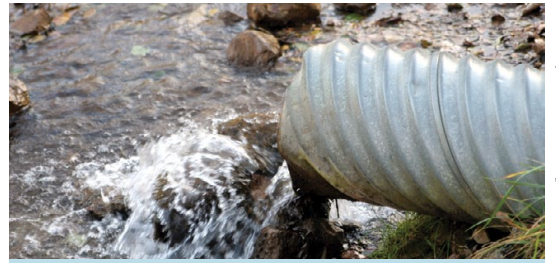
Combined Sewage Overflows threaten communities, especially our beach towns.
