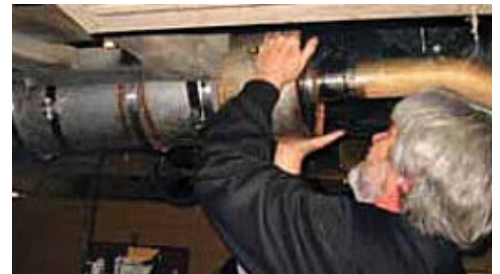
Installation of Diesel Particulate Filters means better health and more Michigan jobs.
